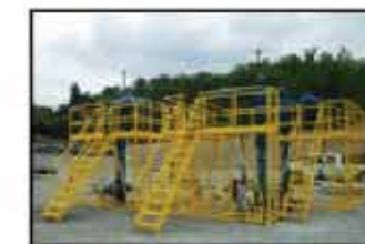
Well Head Access Platforms
